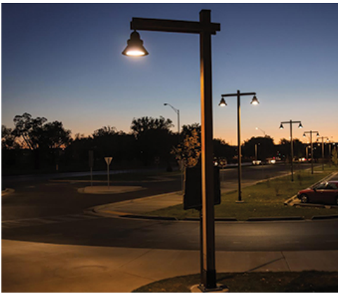
Full cut-off lighting illuminating parking and pedestrian connection. (Credit: landscapeonline.com)
