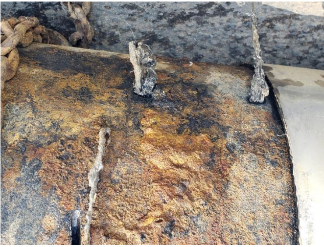
Figure 1 corrosion plugged by rags
