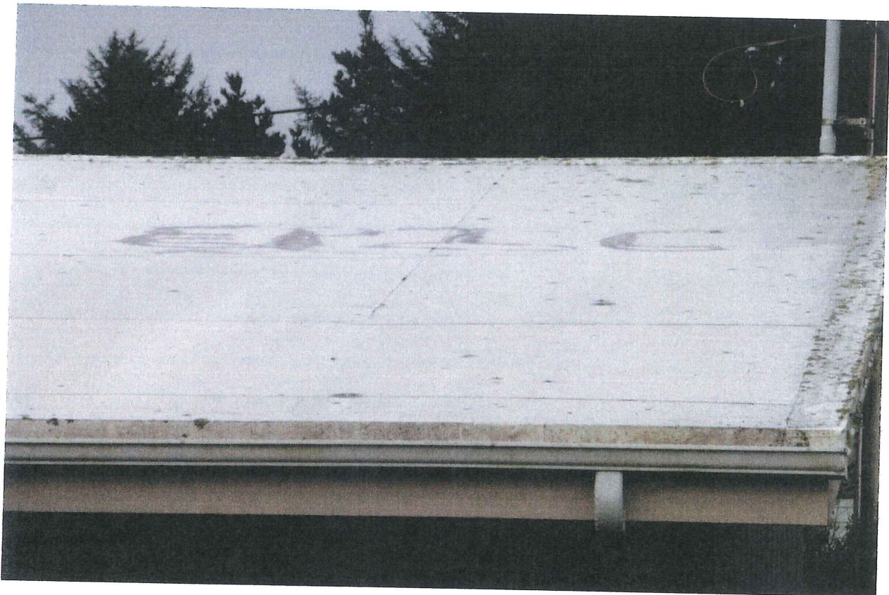
East section of the church, showing graffiti on the roof and how dirty and unsightly it is.
