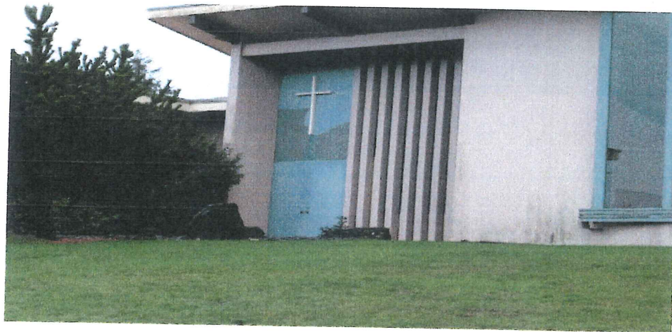
Damage above door.
