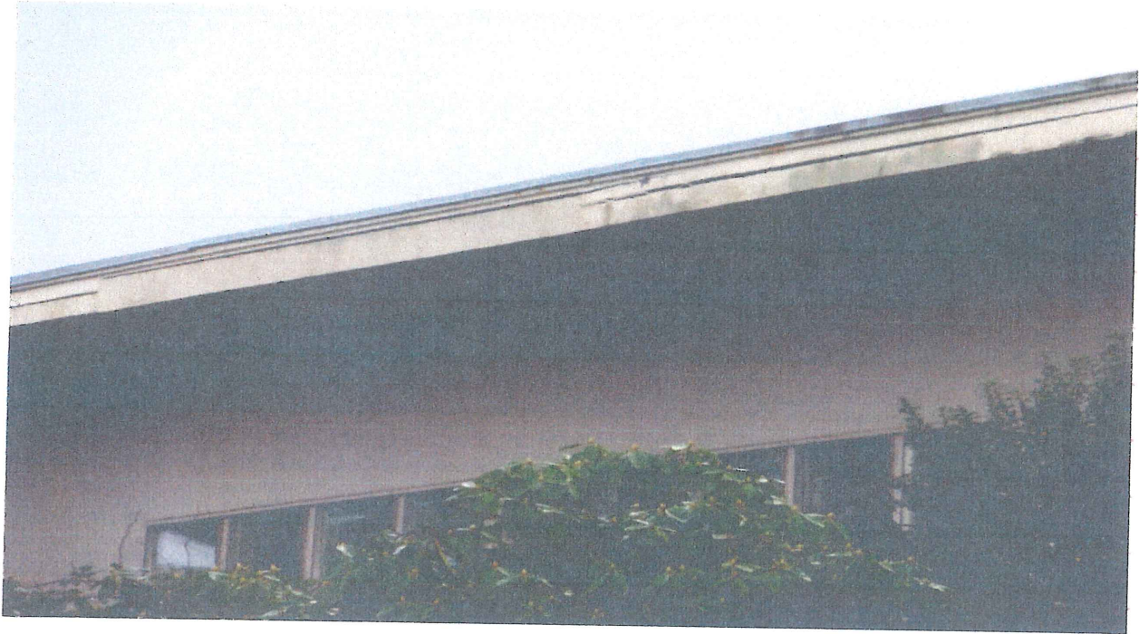
Damage on fascia boards.
