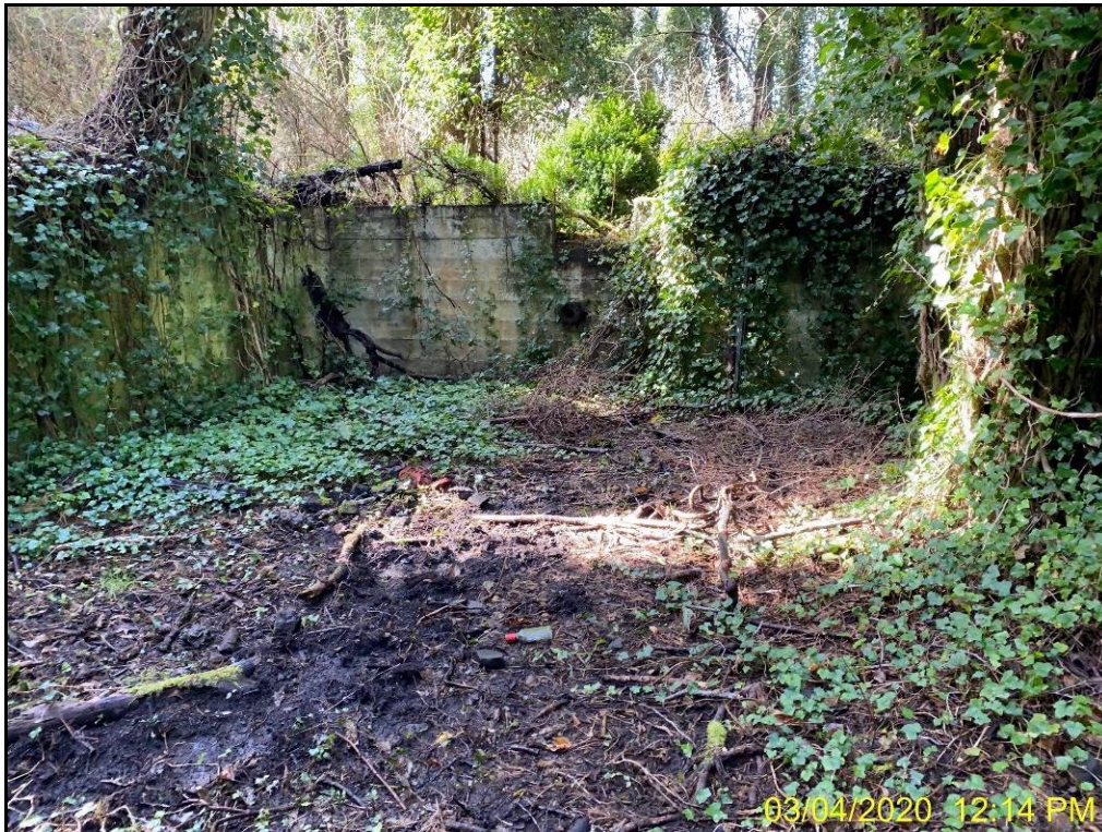
Photo 7: Retaining wall with a large drain pipe near where old residence had been.
