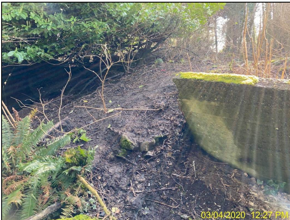
Photo 8: Looking southeast at failed retaining wall near where driveway had entered property from the west.
